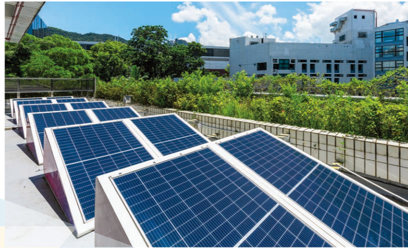
Nearly 2,000 bifacial solar panels will be installed on the rooftops of over 30 campus buildings. 城大將在校園內30多幢建築物天台上，安裝近2,000塊雙面太陽能板。
